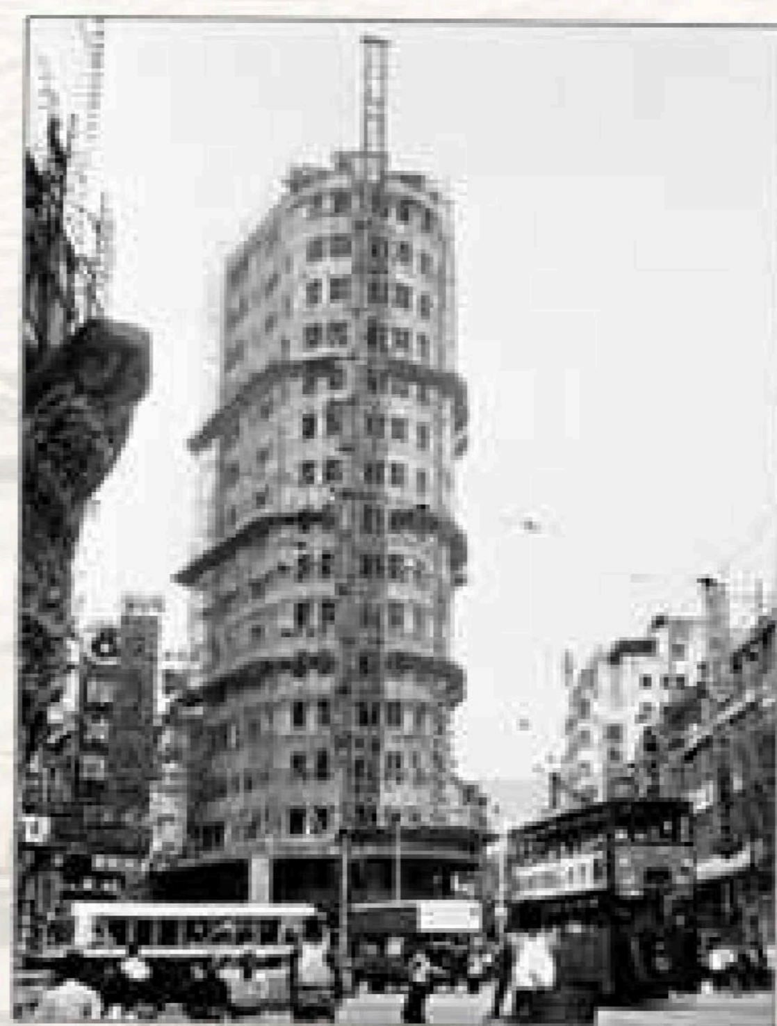
New building under construction at the junction of Johnston Road and Wan Chai Road (1963)
